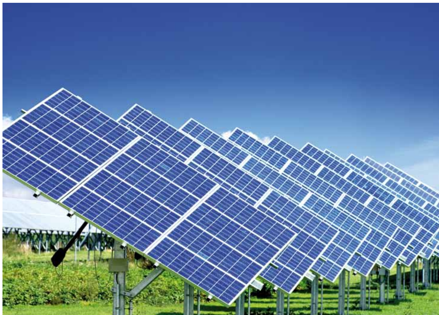
Photo: Solar plant on open land
